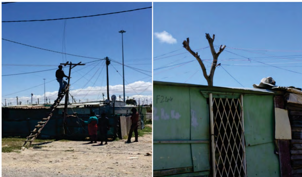
Figure 2-3: A view an informal areas showing various electrical connections that are a significant problem for fire safety
