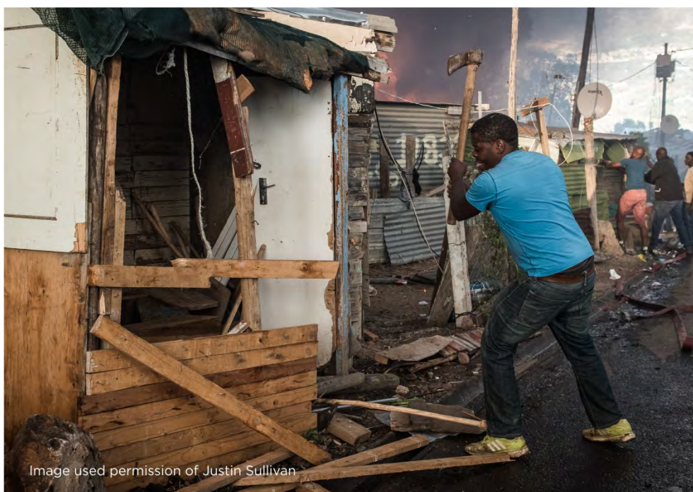
Figure 6-8: Dry firefighting techniques being employed by a resident trying to demolish his home to prevent spread and possibly save the construction materials. (Image used permission of Justin Sullivan)
