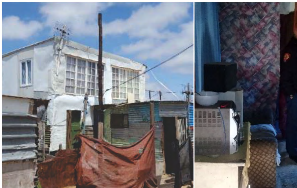
Figure 2-1: (Left) A variety of unregulated construction methods and materials are utilised to build informal dwellings, and (Right) flammable synthetic materials lining a home, positioned against electrical equipment.
